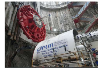
Urban sewerage, Singapore
